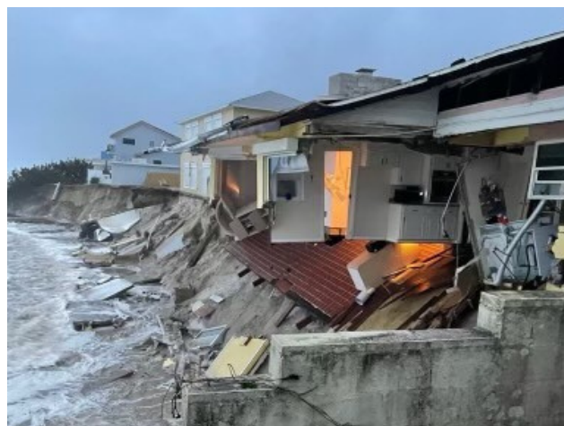
Substantial damage from Hurricanes Ian and Nicole to homes in Wilbur-By-The-Sea, Volusia County
